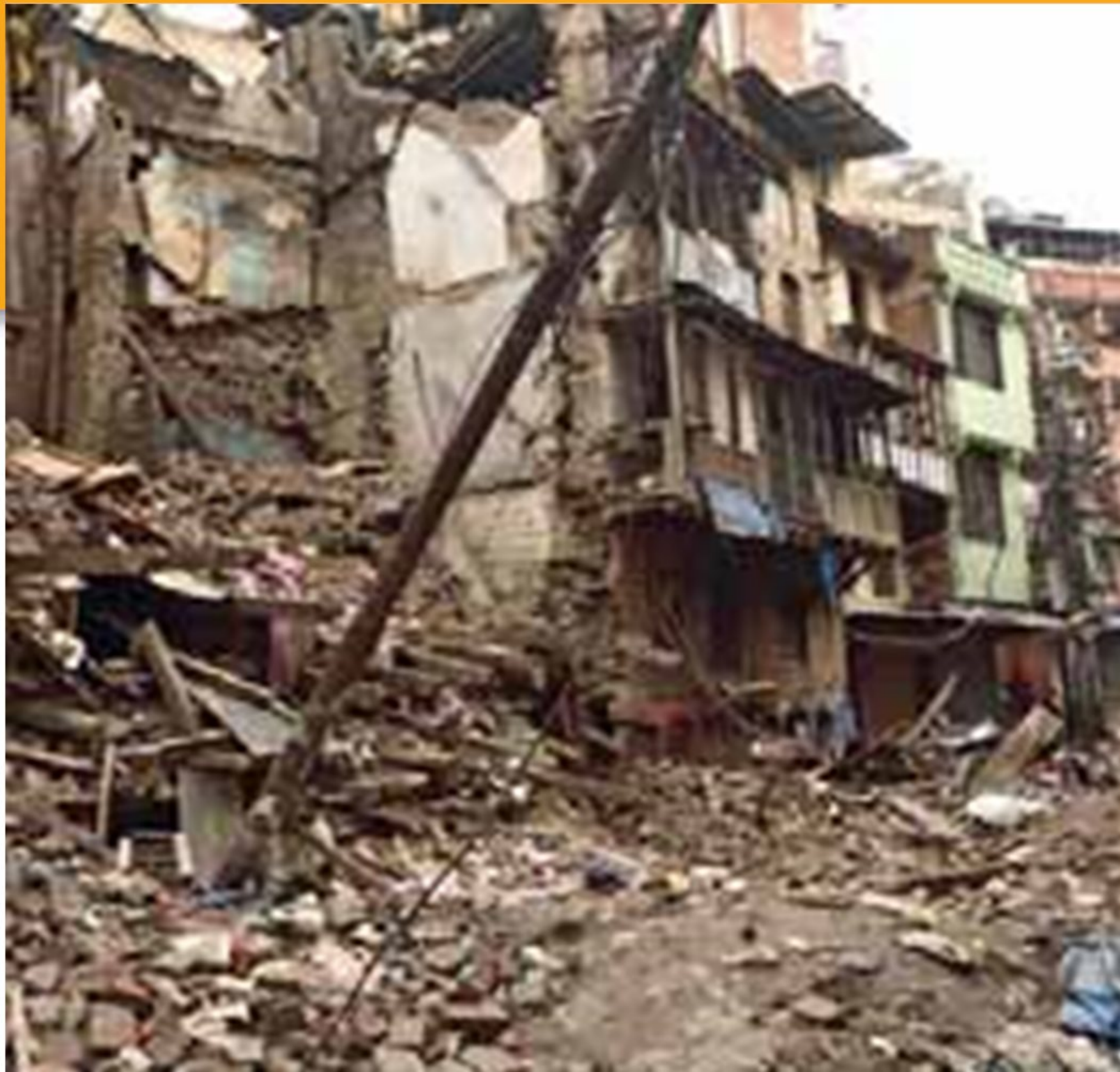
■ Figure 2.1 Earthquake damage in Kathmandu, Nepal, 2015
